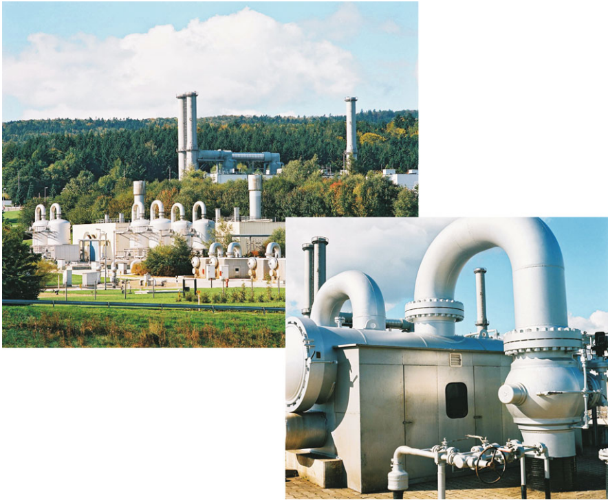
Fig. 8 Compressor (source: E.ON Ruhrgas)
