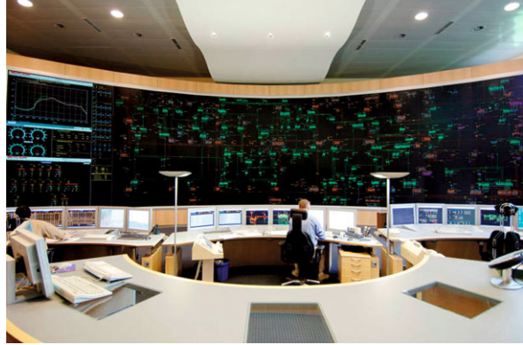
Fig. 2 Control center of a large transmission grid operator (source: RWE)
